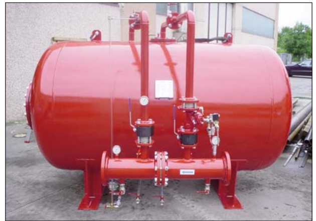
Figure 3. Horizontal bladder tank
